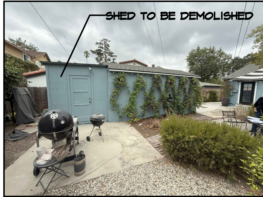
NORTH ELEVATION OF GARAGE AND PLYWOOD SHED BUILT WITHOUT PERMIT IN 1995.
