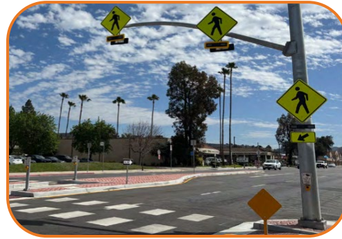
Rectangular Rapid Flashing Beacon
