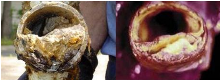
A clogged sewer
